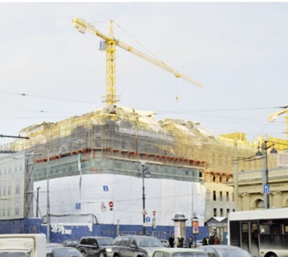
The Nevsky Centre shopping centre and department store under construction in St Petersburg is impressively large. The site covers one hectare and, upon completion, the retail space will equal that of the enlarged Stockmann department store in the centre of Helsinki.
